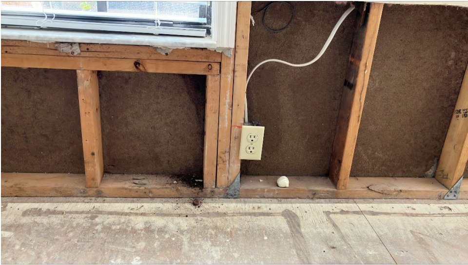
Water damage in sheathing dining room area
