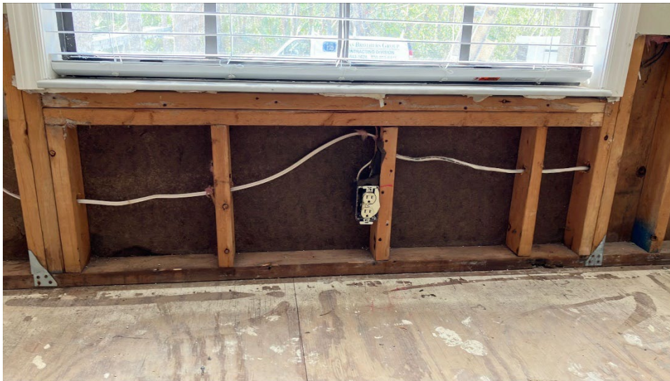
Wood sheathing has water damage
