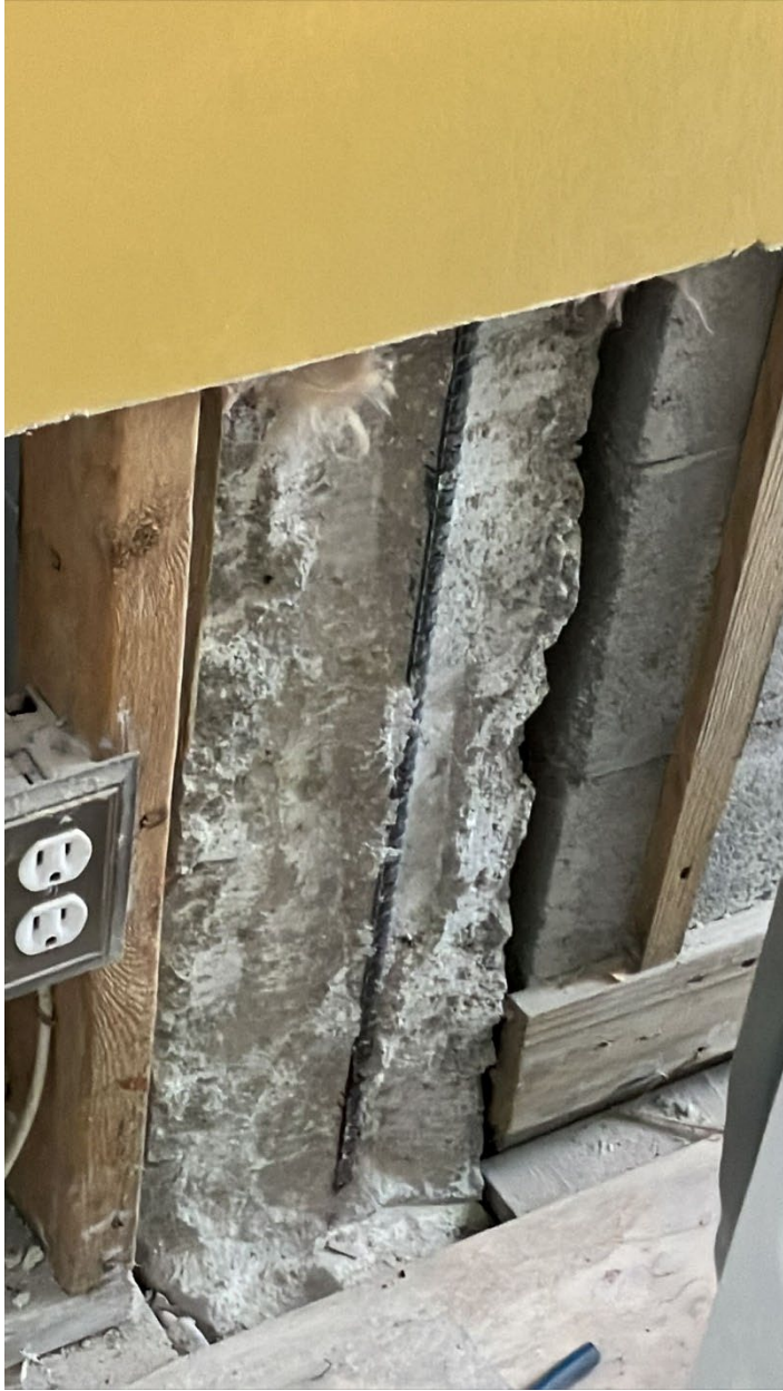
Exposed rebar in kitchen column ??
