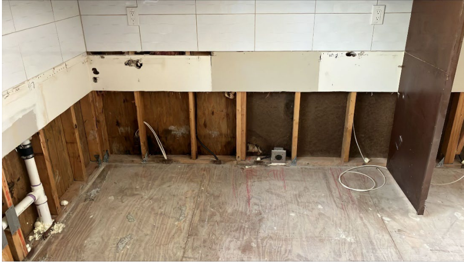
Kitchen, rotten wood sheeting
