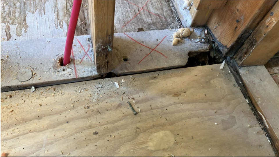
Completely rotted to 2x4 Frames and subfloor
