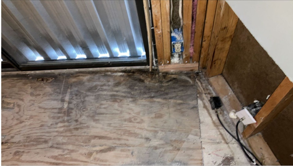
Master bedroom right side of sliding glass door, subfloor rotting
