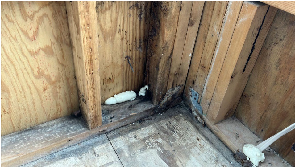
Dining room area, rotting subfloor
