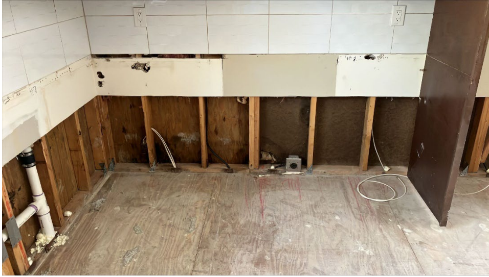
Kitchen, rotten wood sheeting
