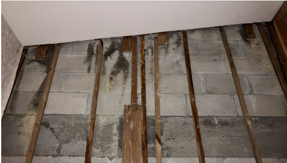
Master bathroom, potentially mold on cinder blocks
