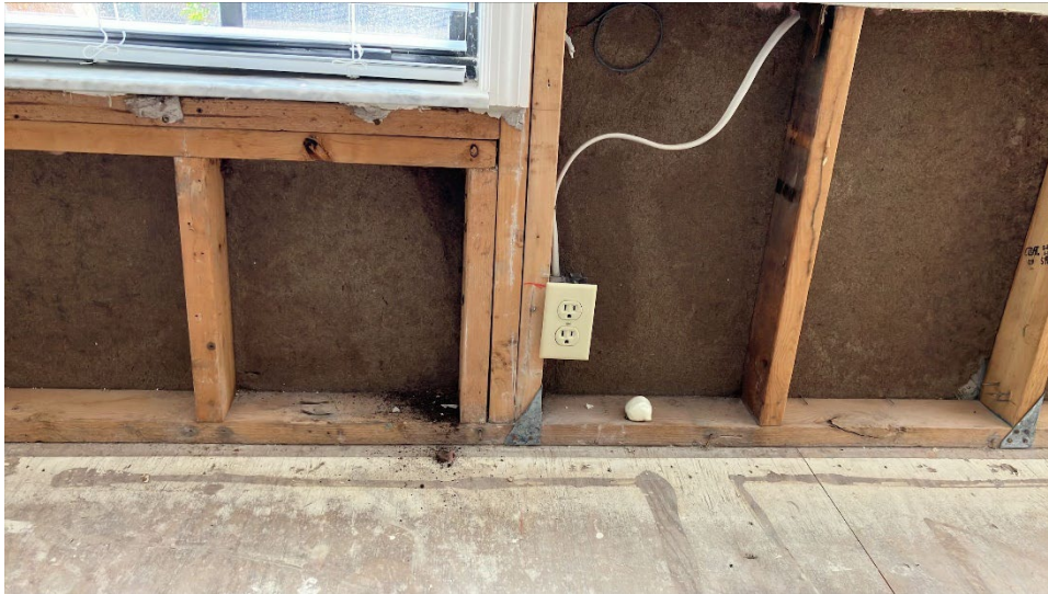
Water damage in sheathing dining room area
