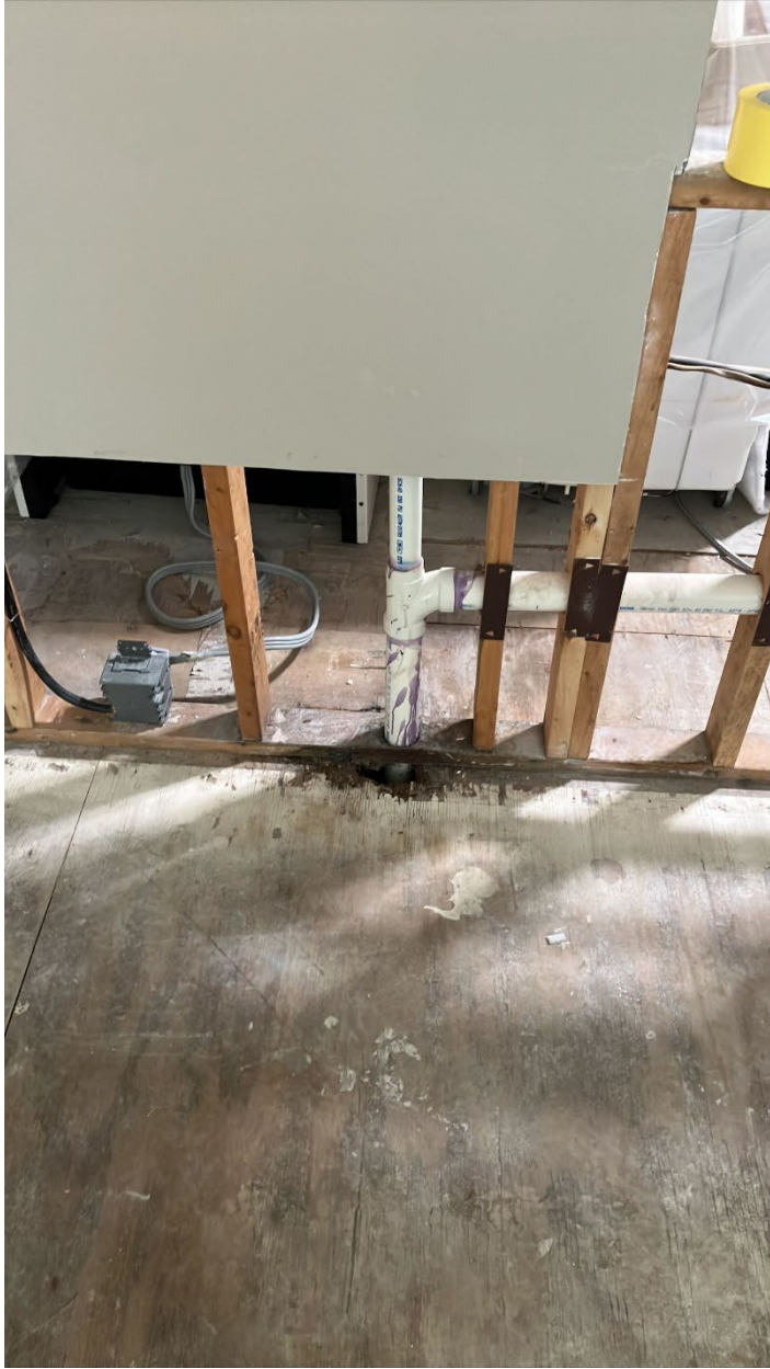
Back side of sink wall facing the living room there is floor rotting
