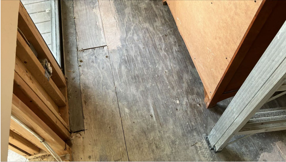
MBR sub floor?
