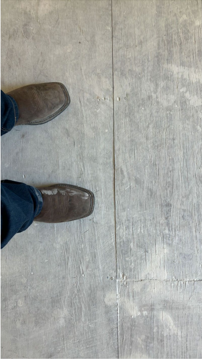
Subfloor in guest bedroom loose
