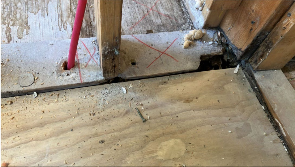
Completely rotted to 2x4 Frames and subfloor
