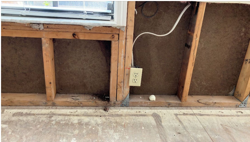
Water damage in sheathing dining room area
