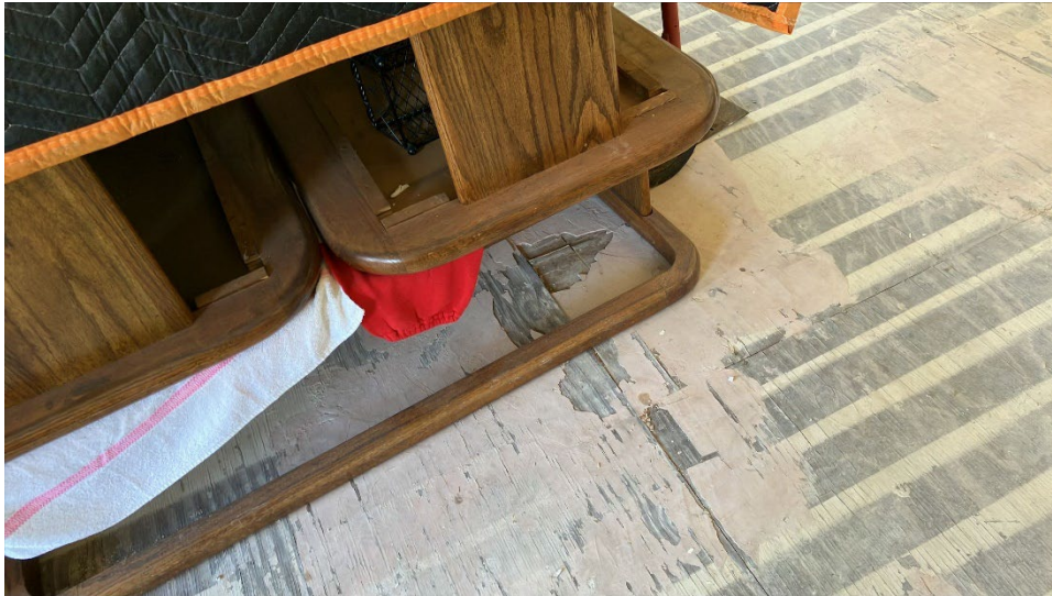
Living room area subfloor ?
