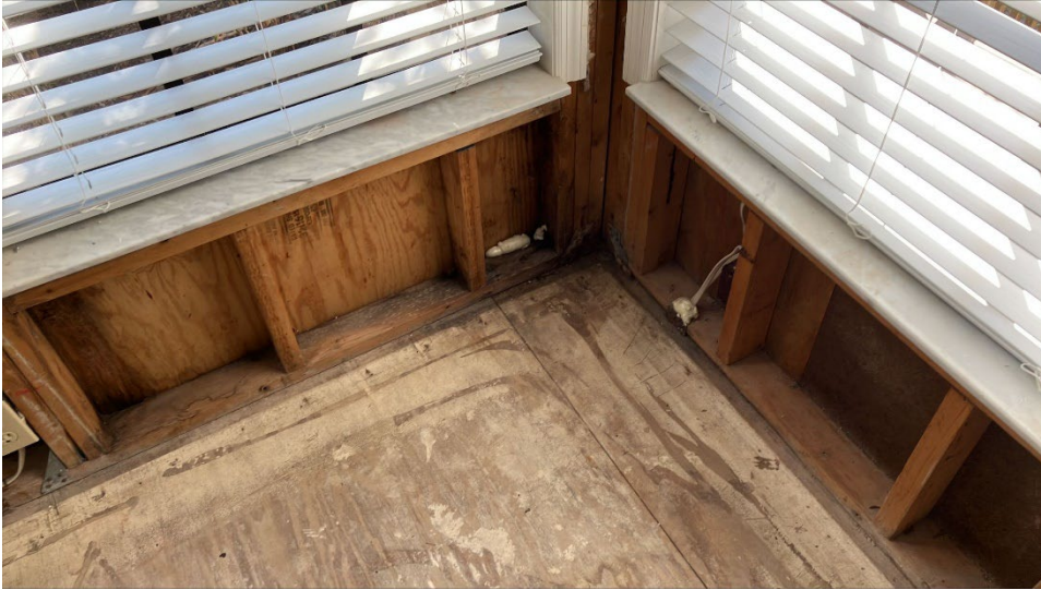
Dining room area, rotted, framing
