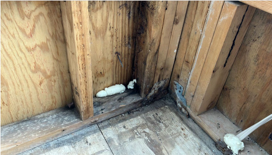
Dining room area, rotting subfloor
