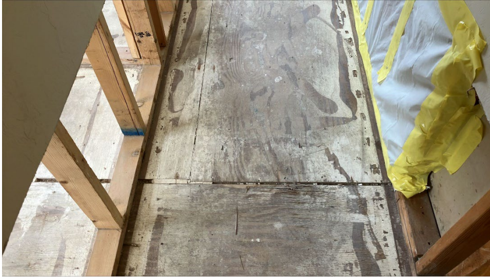
Hallway, rotted, wood, subfloor
